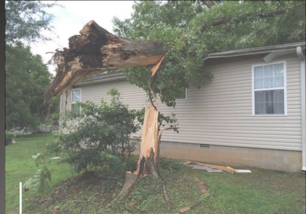
Tree damaging your house
