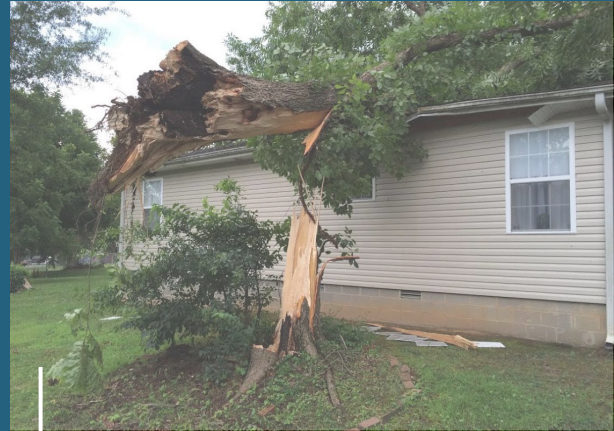
Tree damaging your house
